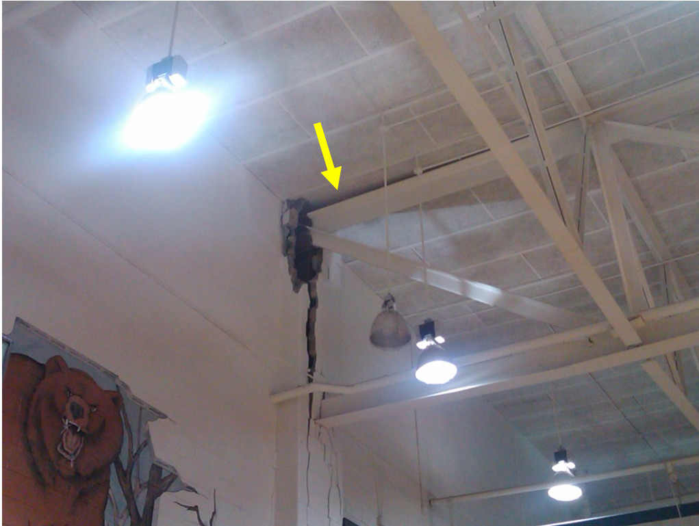
Figure 1: Cell phone picture taken during roof failure shows separation between the top member of the truss and the roof (arrow) on the southwest side.
