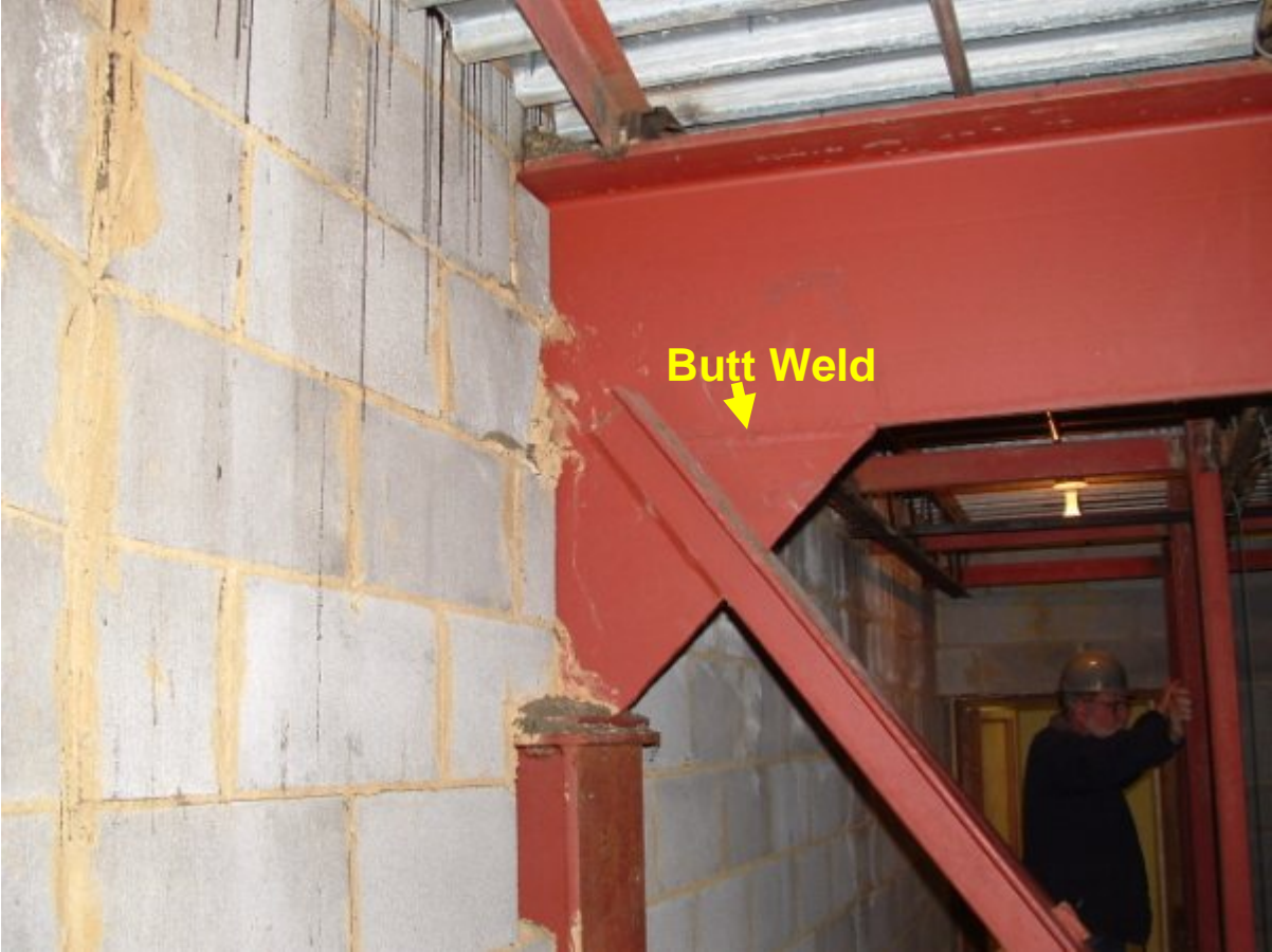
Figure 3: Truss in auditorium illustrates construction geometry. This support uses the same design as the gym roof support but is smaller.
