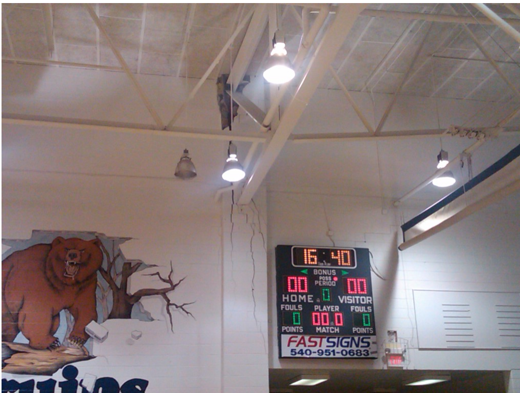
Figure 2: Cell phone picture taken during roof collapse shows southwest side top member pulling to the left side of the column, compared to the bottom member which was located in the center of the column.
