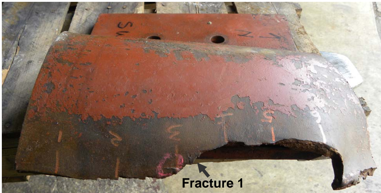
Figure 4: Base section of support after fracture. Note how web has collapsed onto base. (Note: photos, when appropriate, have been rotated to match original as-constructed orientation).
