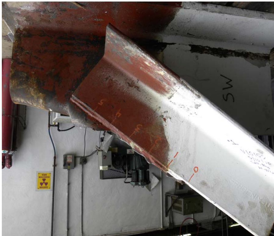
Figure 7: Top truss member as viewed from the sides. Arrows point to Fracture 2 on weld.
