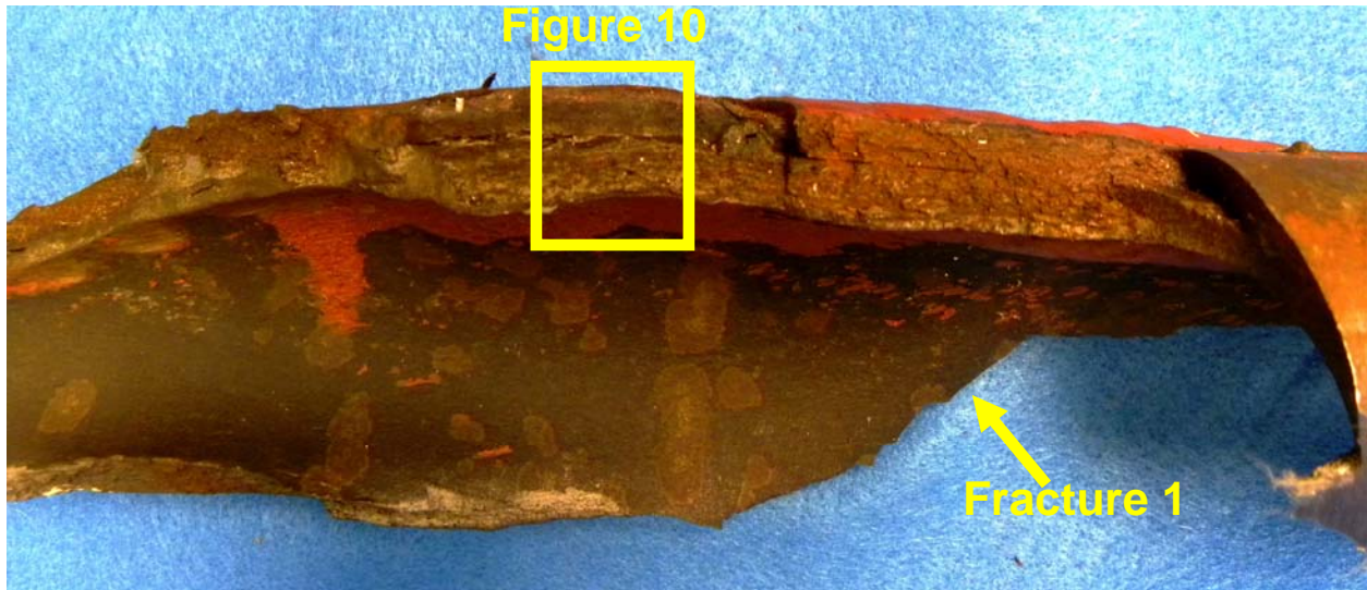
Figure 8: Closer views of Fracture 2. Note “ridge line” in center of fracture in bottom photo.
